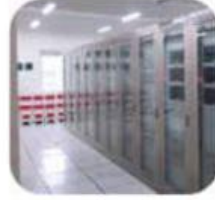
继保室 Relay Protection Room
